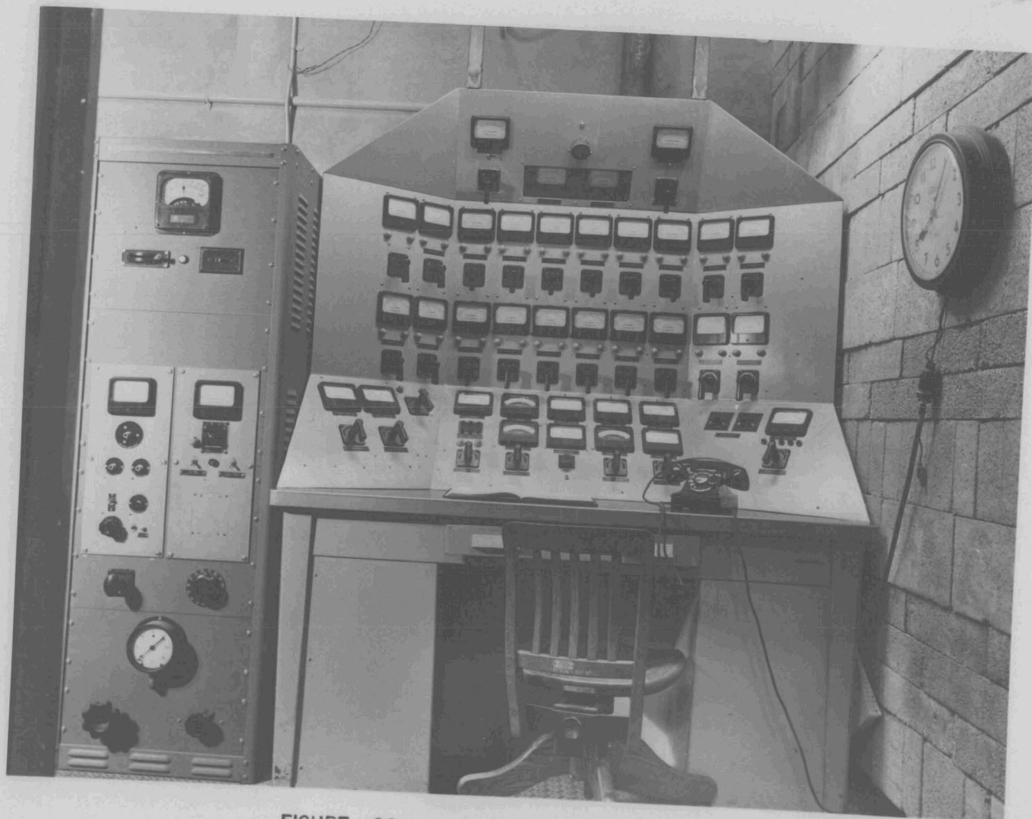
FIGURE 29. LOCAL CONTROL STATION
